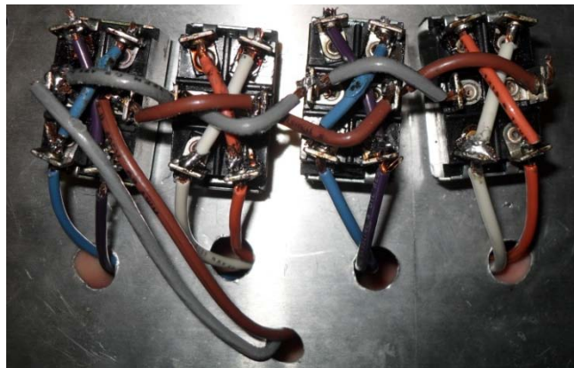
Figure 41: The switchbox wiring.
